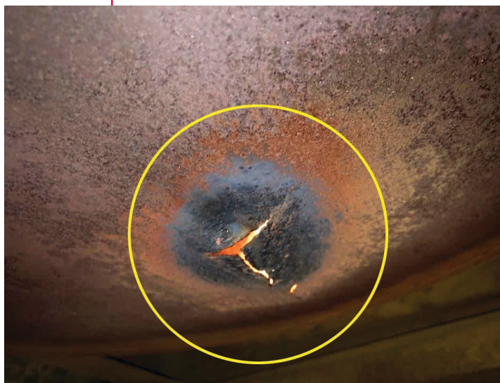
Figure 13-9: Visible defect to show customer
