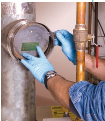
Adjusting draft regulator on flue
