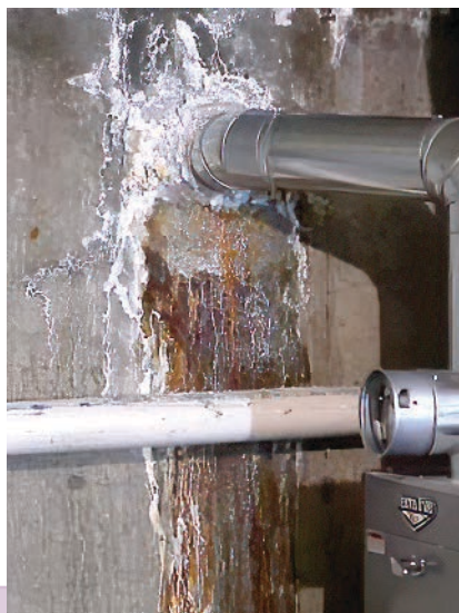
Figure 15-2: Evidence of water coming down chimney
