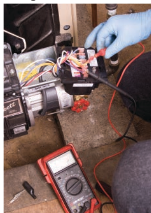
Using an electrical meter
