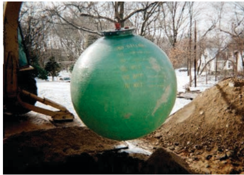
Figure 3-15: Fiberglass (FRP) tank
