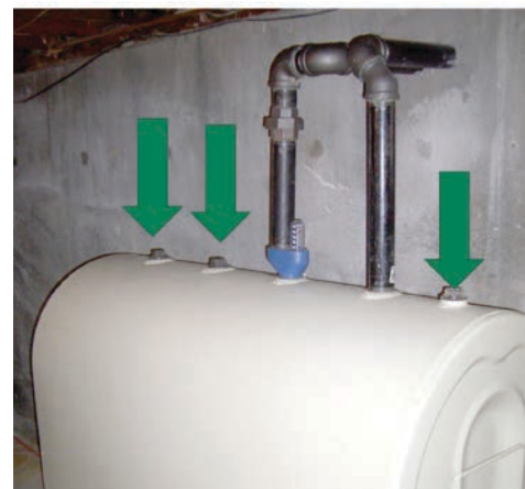
Figure 3-20: Unused tank openings must be plugged with threaded steel plugs
