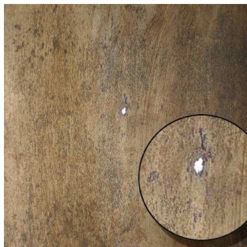
Figure 3-2: Internal corrosion with pin hole magnified
