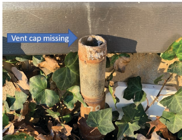
Figure 3-3: Missing vent cap may be a source of water in the tank
