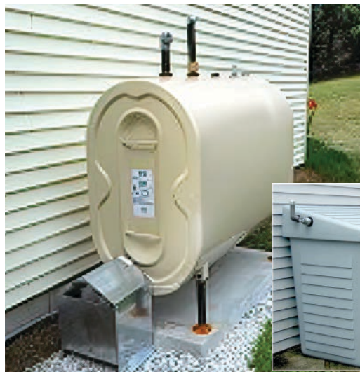
Figure 3-5: Outside above ground tank. NORA recommends painting outdoor tanks a light color to reduce extreme temperature swings. Inset: tank enclosure
