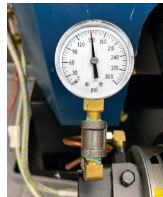
Figure 4-13: Fuel unit at 150 PSI
