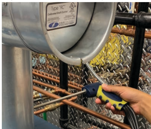
Checking composition & temperature of the flue gases at the breech
