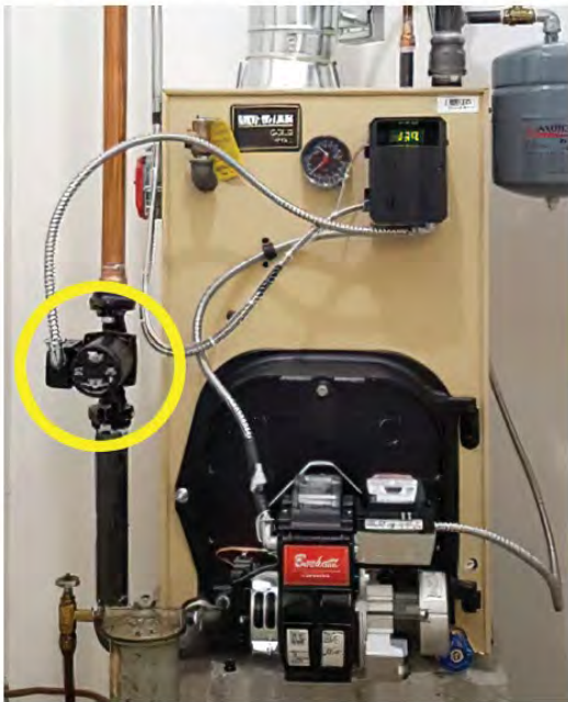
Figure 13-20: Circulator located on return line
