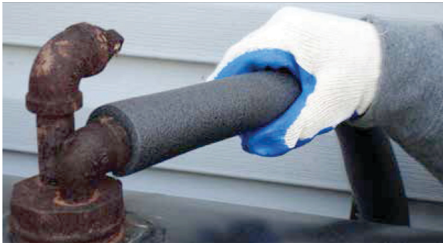
The fuel line to the house is insulated, but the piping could benefit from some rustproofing paint.
